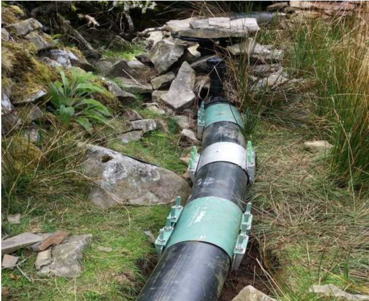
Photo: Repaired penstock with new clamp near the intake of Nant yr Hafod
