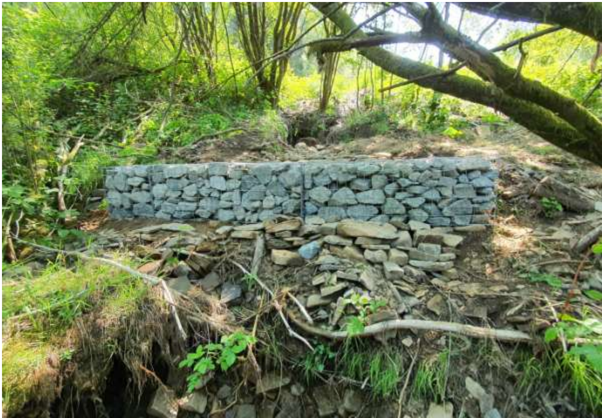
Photo: New gabions filled with stone to support the penstock pipe at Cwm Saerbren
